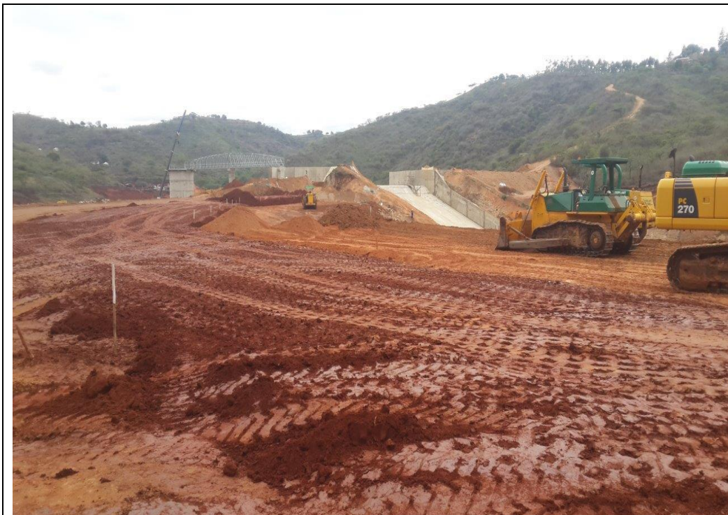
Invutshane Dam nearing completion near Stanger, Owner: Umgeni Water (H = 28 m, V = 3,1 million m 3 , category II)
